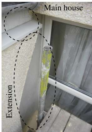
Figure 1: Example of thermal bridging resulting from an inadequate preliminary survey
