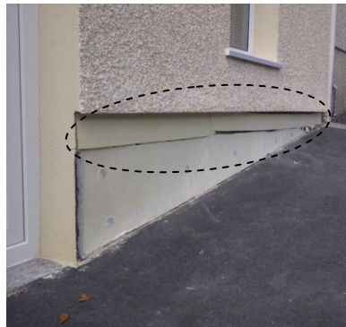
Figure 2: Example of poor execution, which could lead to thermal bridging
