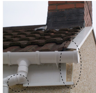
Figure 3: Example of poor detailing and execution resulting from an inadequate preliminary survey
